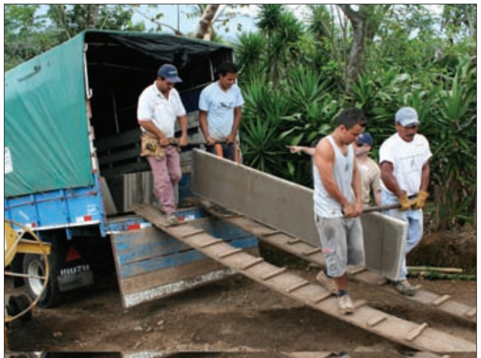
Luis (from left), Leo, Bennicio and Eliezer carry a 500-pound cement block that will become part of a wall off the delivery truck.
